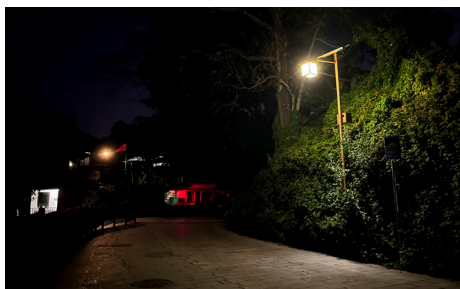
The lighting effect of the pole light
